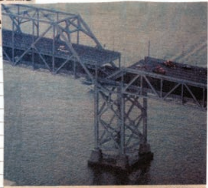
An aerial view of the collapsed bridge roadway
